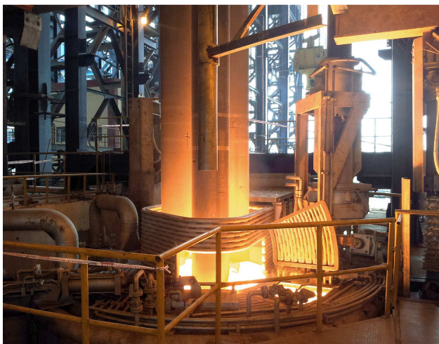
The new 250-ton ladle furnace.
