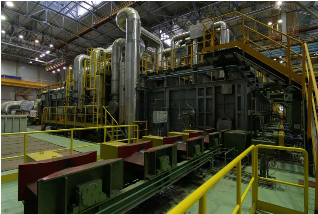
The walking beam furnace for PT. Gunung Raja Paksi, which will be similar to the one shown here, will be equipped with SMS Prometheus software to achieve excellent heat efficiency.
