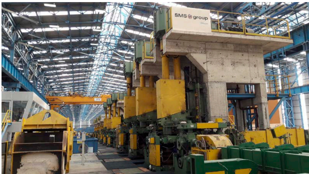
PT. Gunung Raja Paksi's rolling mill, similar to the type shown here, will be designed for an annual production of 500,000 tons.
