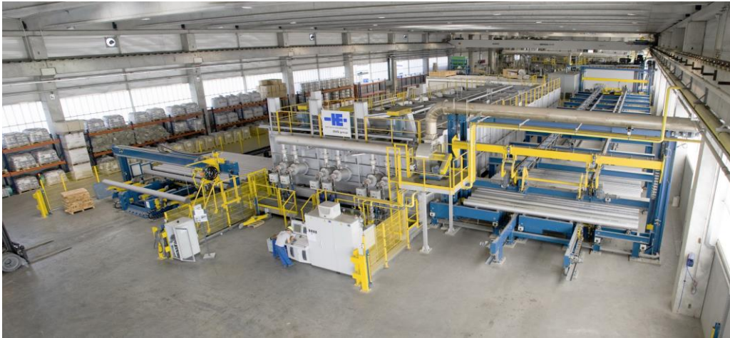
Existing continuous homogenizing plant at Hammerer Aluminium in Romania.
