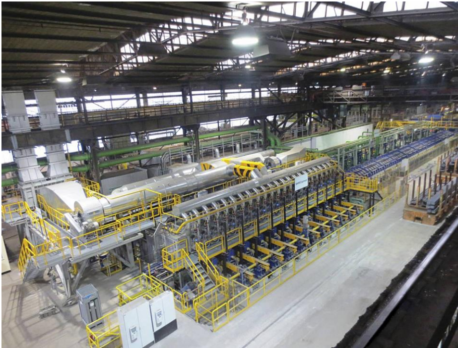
New heating concept to make production more energy-efficient and climate-friendly.
