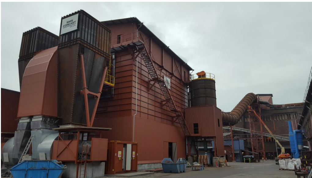
Fan configuration and stack design with reduced chimney dimension. The high-performance filter from SMS group requires less energy.
