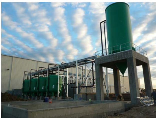
SMS group's scope of supply also includes the water treatment plant.
