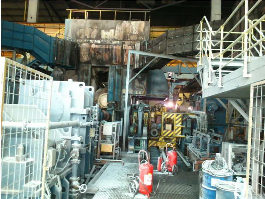
Rolling stand immediately after the fire.
