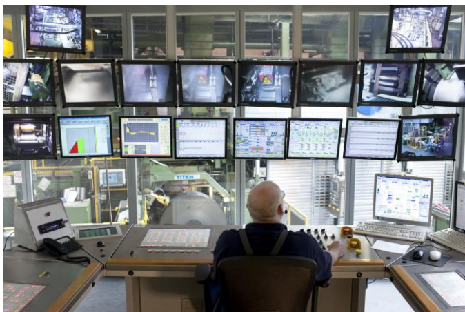
View to the control room.
