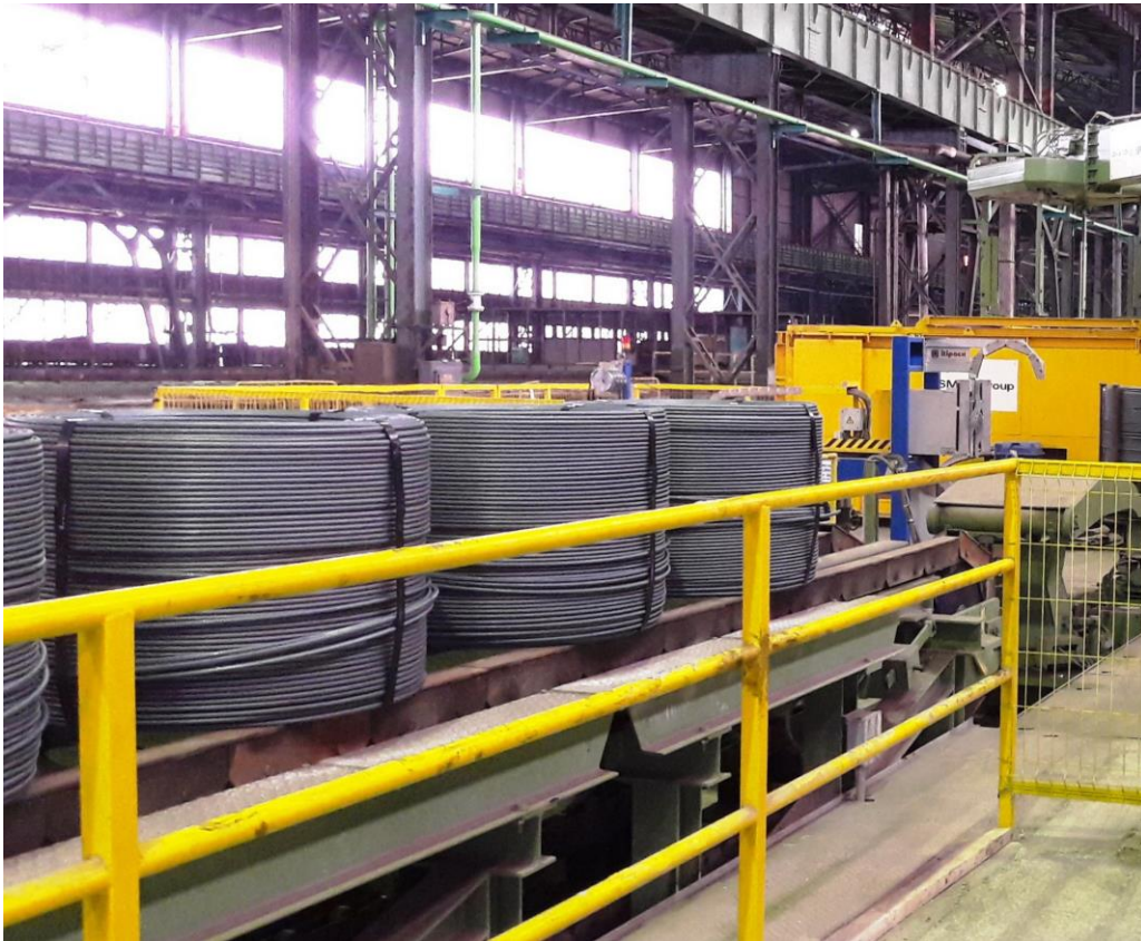
The new VCC ® line (Vertical Compact Coiler) at ArcelorMittal Zenica d.o.o., Bosnia and Herzegovina, which operates at a throughput of 60 tons per hour.
