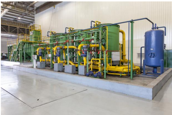
Example of a rolling-oil treatment plant using a SUPAFINE ® filter system.
