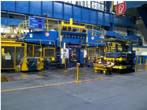
Ready for new tasks: the SMS 20-roll cold rolling mill at Outokumpu Nirosta GmbH Krefeld.
