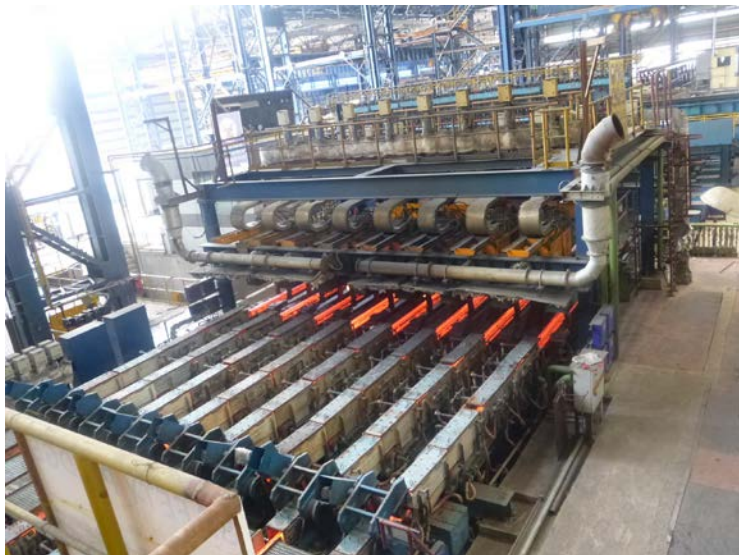
High-speed eight-strand billet caster at JSPL Angul Odisha plant.
