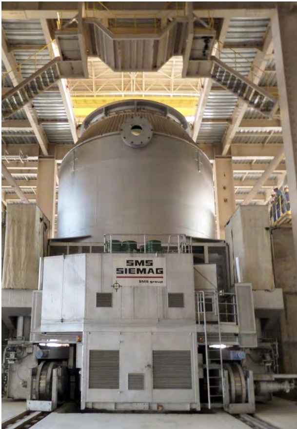
The converter vessel-changing car from SMS Siemag has a working load of 1,200 tons.
