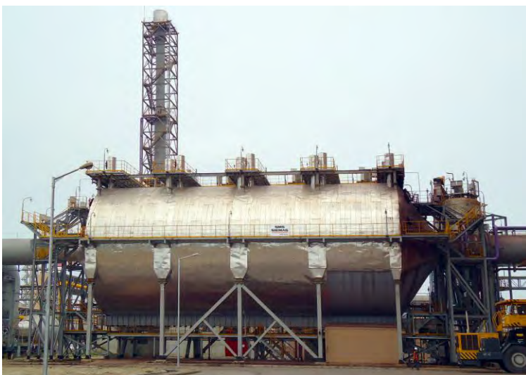
Highly effective environmental technology with the dry-type converter-gas dedusting system from SMS Siemag.
