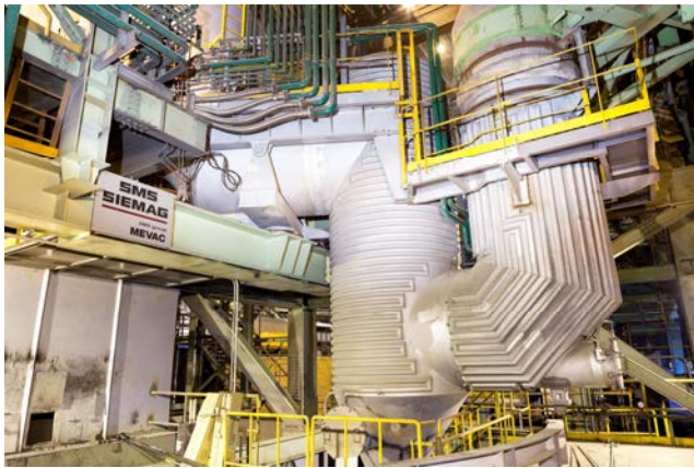
The RH plant No. 8 has a modern gas cooler.
